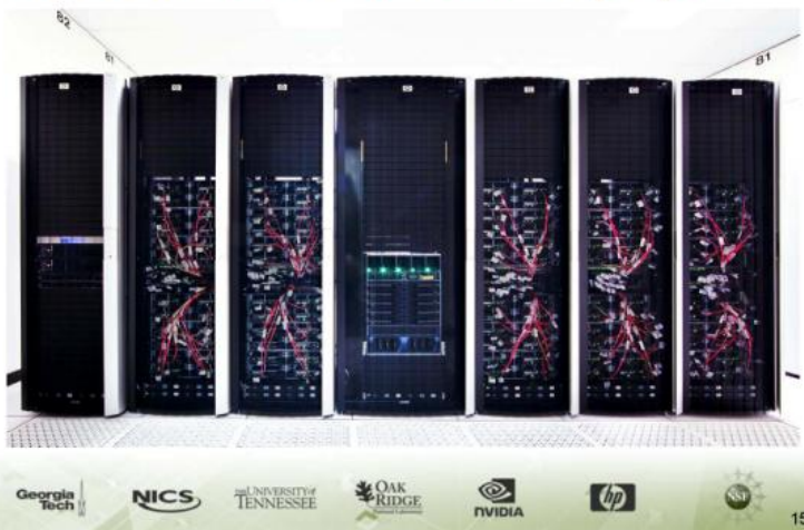
Keeneland ID installation – 10/29/10
